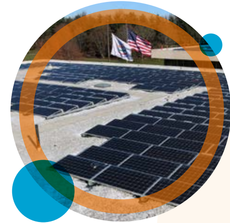
PepsiCo recently installed new solar rooftop panels on our New York global headquarters.
